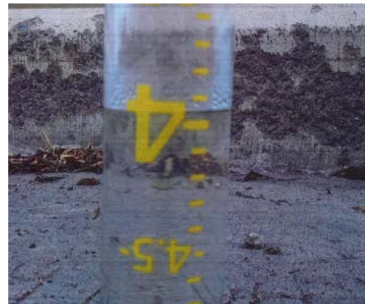
Untreated bridge deck showing water
